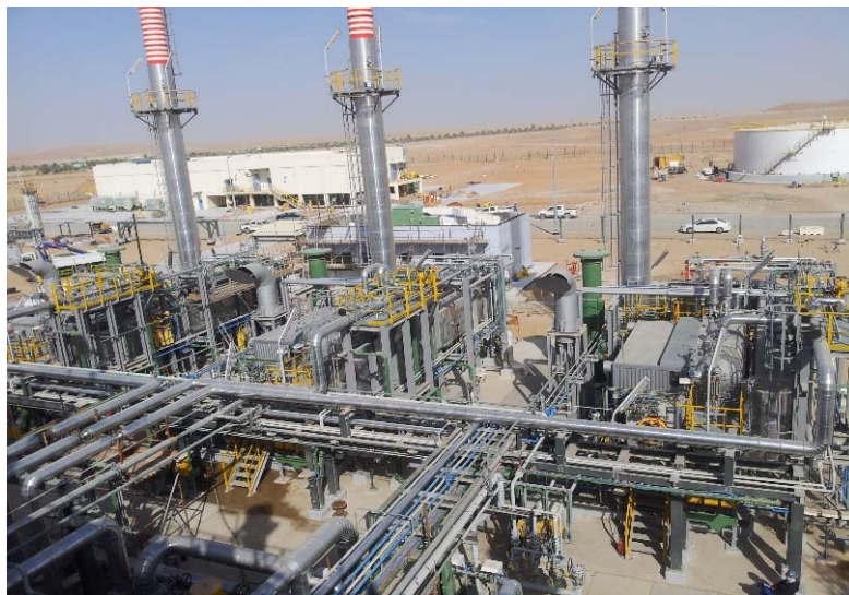
WATER TUBE BOILER - GASCO HSGP PROJECT, U.A.E.
