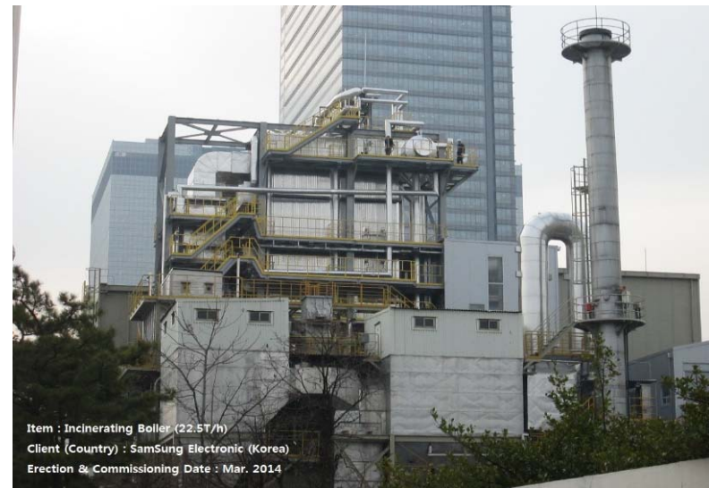
ICW WASTE HEAT BOILER - SAMSUNG ELECTRONICS CO., S. KOREA
